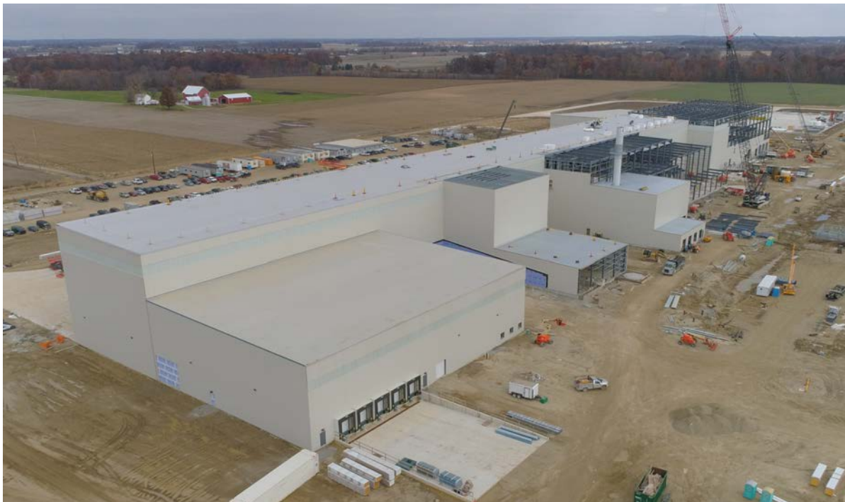
Pratt Industries' latest Midwest investment under construction is the Wapakoneta millugator in Ohio (Photo: Supplied)
