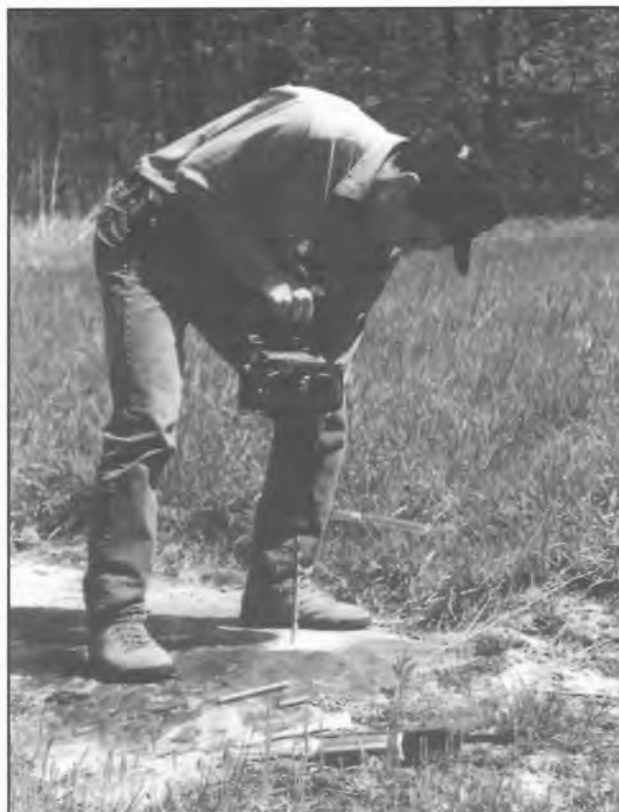
DIGGING IT: Mike Hamburger drills a hole for a geodetic benchmark used in the Wabash Valley.
